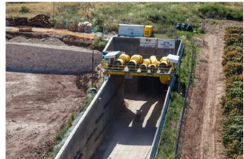
Ventilation System in MAT Portal
